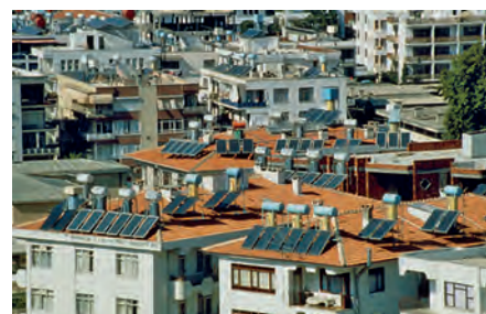
Solar heating panels on top of houses in Antalya. The position of solar panels depends on the amount and direction of sunlight as well as the design of the building and other considerations.
